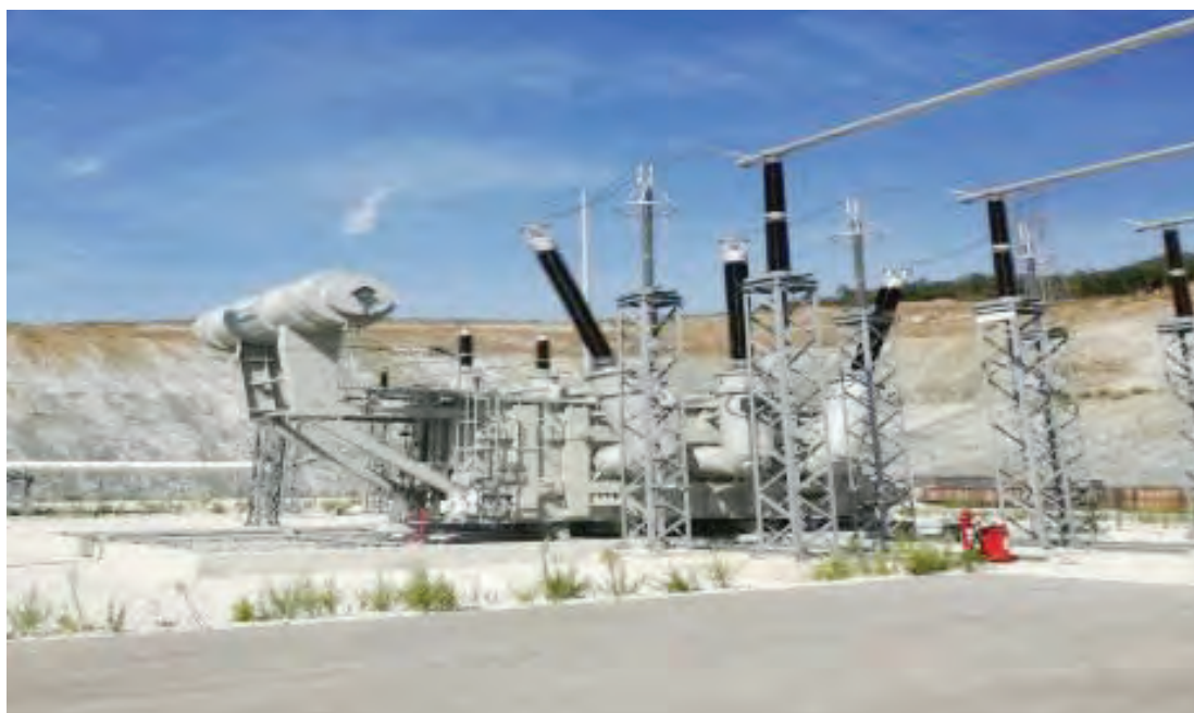
Figure 15. Power transformer 300MVA 400/110/10.5 kV
