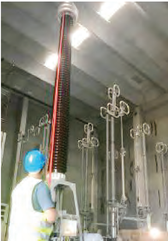
Figure 9 - Final checks to the cable termination and generator before the 700kV test on the complete MONITA HVDC cable system in the DC hall of the Converter Stations of Kotor (MNE).
