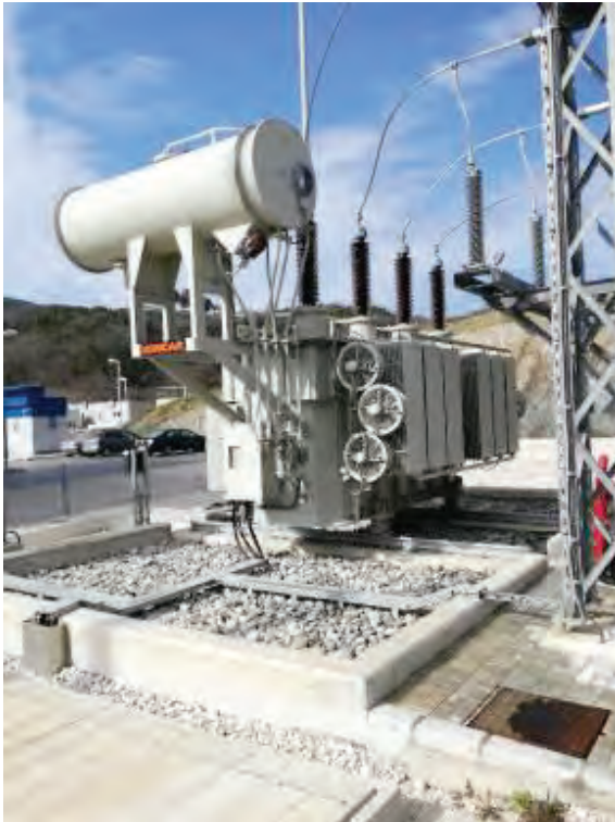
Figure 17. Power Transformer 110/36.75/10.5 kV 20MVA
