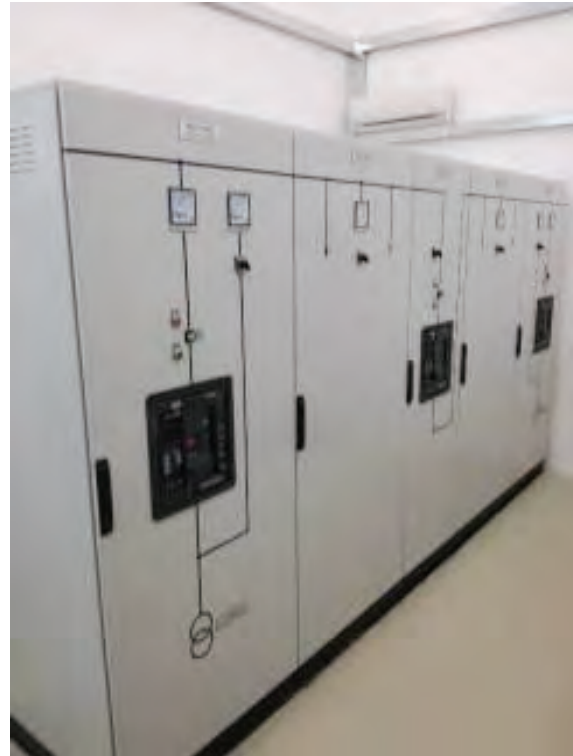
Figure 18. Main Supply Cubicles in SS Lastva AC/DC room
